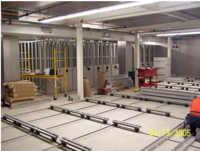
Workers prepare new vaults at the National Audio-Visual Conservation Center in Culpeper, Virginia. (photo courtesy LC)
